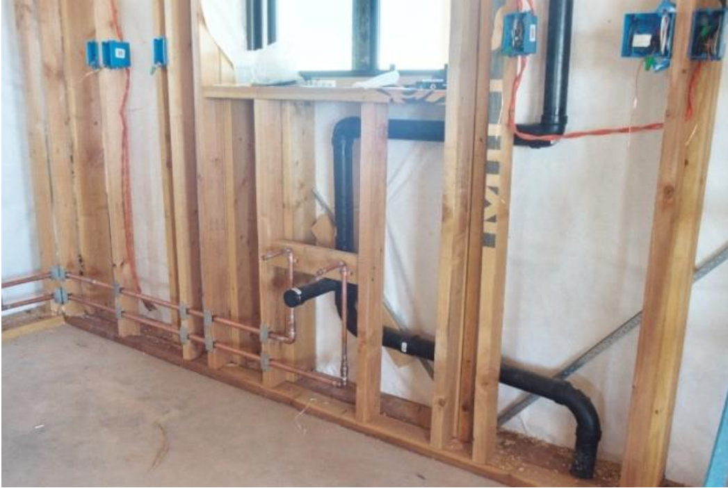
Outer wall with redwood bottom plate, Douglas fir studs, housewrap and plumbing. Insulation and drywall came later.
