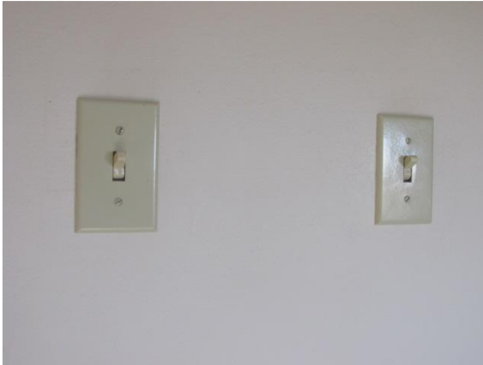
A kill switch (left) and a regular light switch near a door to a bedroom.
