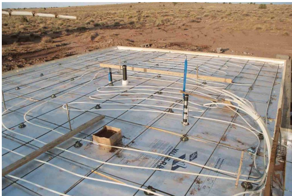
Even better are in-floor heating systems, which can be designed to be completely noiseless and zero-EMF.
