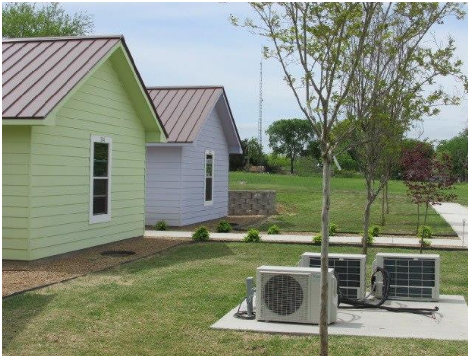
Heating and cooling using a mini-split heat pump located away from the house.
