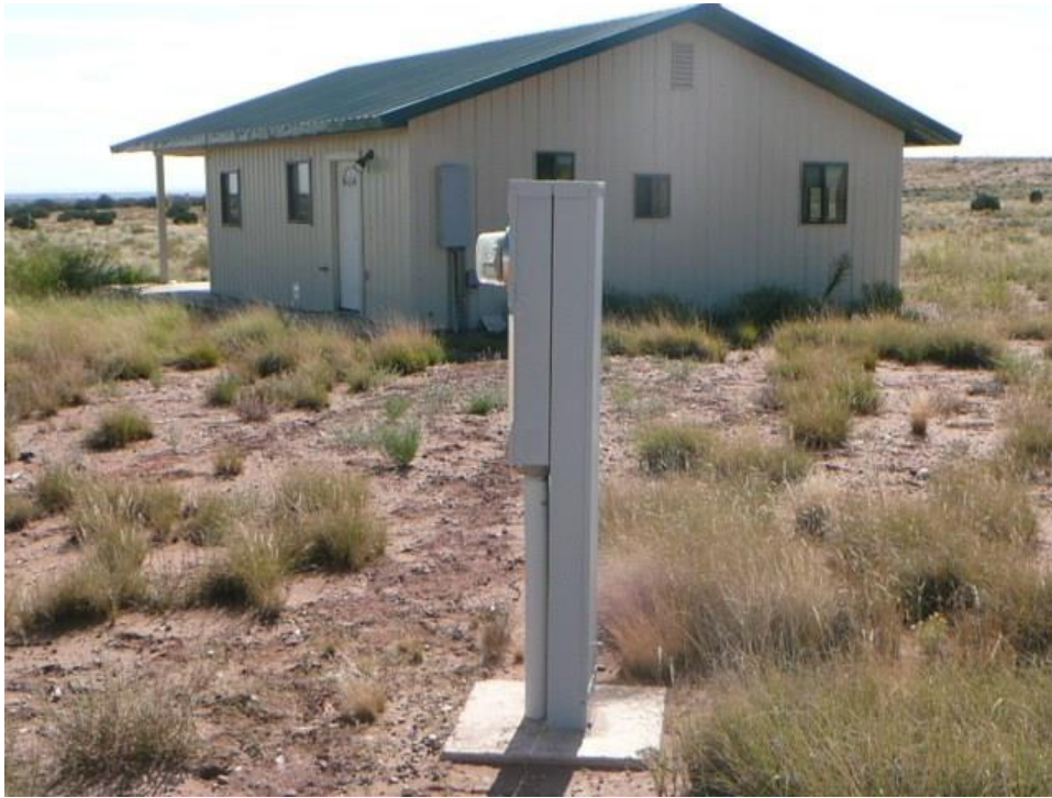
Placing the electrical meter on a pedestal away from the house helps with wireless smart meters. Most of the radiation comes out the front, so it should not point towards the house.
